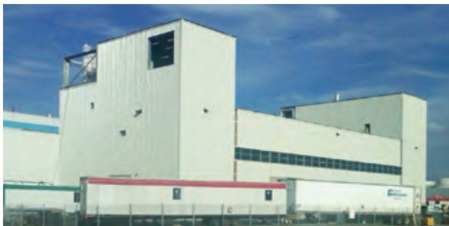
NCC will be produced in a 35,000 sq ft commercial demonstration plant currently under construction on the site of Domtar's pulp and paper mill in Windsor, Quebec, Canada
